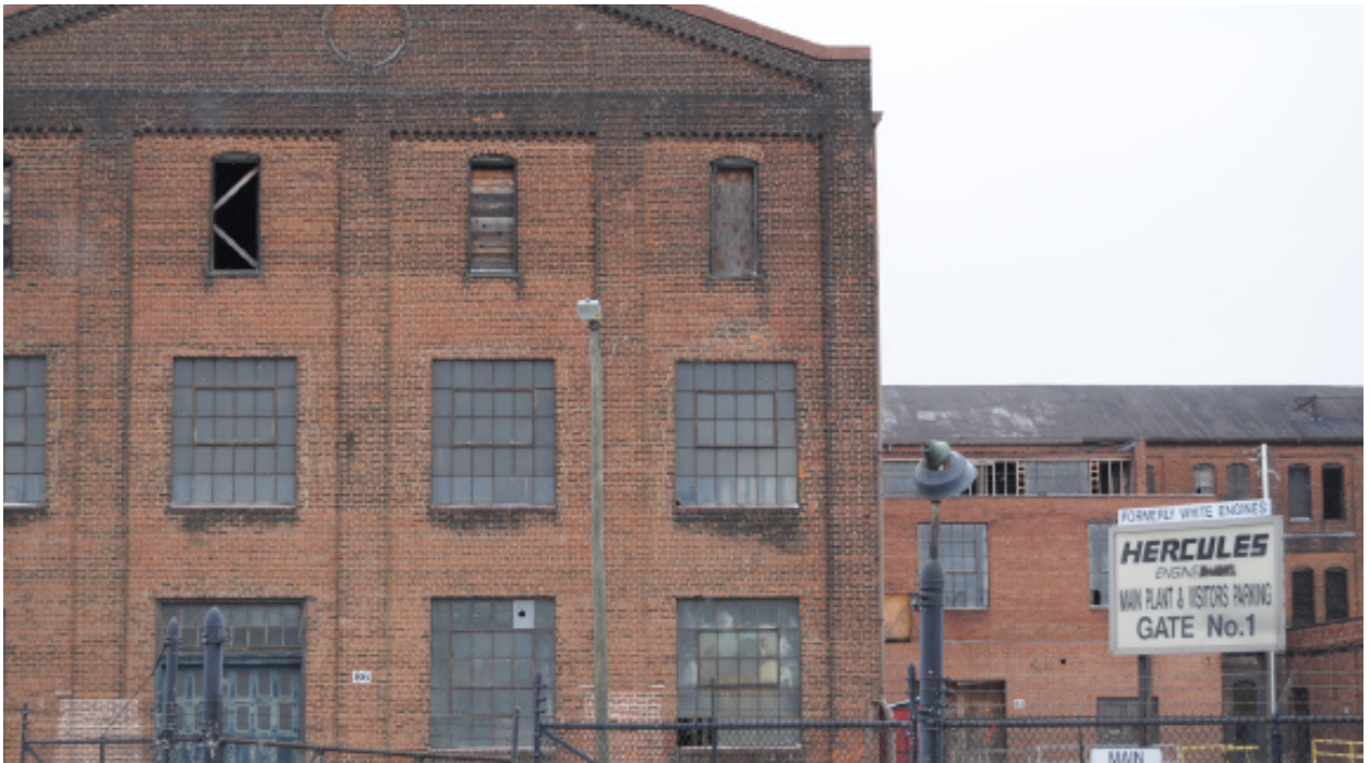
Figure 15: Existing view depicting the physical condition of the existing structure from the exterior
